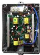
Battery back up with fan cooling systems
