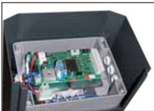
Electronic control unit positioned on the top of the carter
