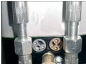
By pass valves
